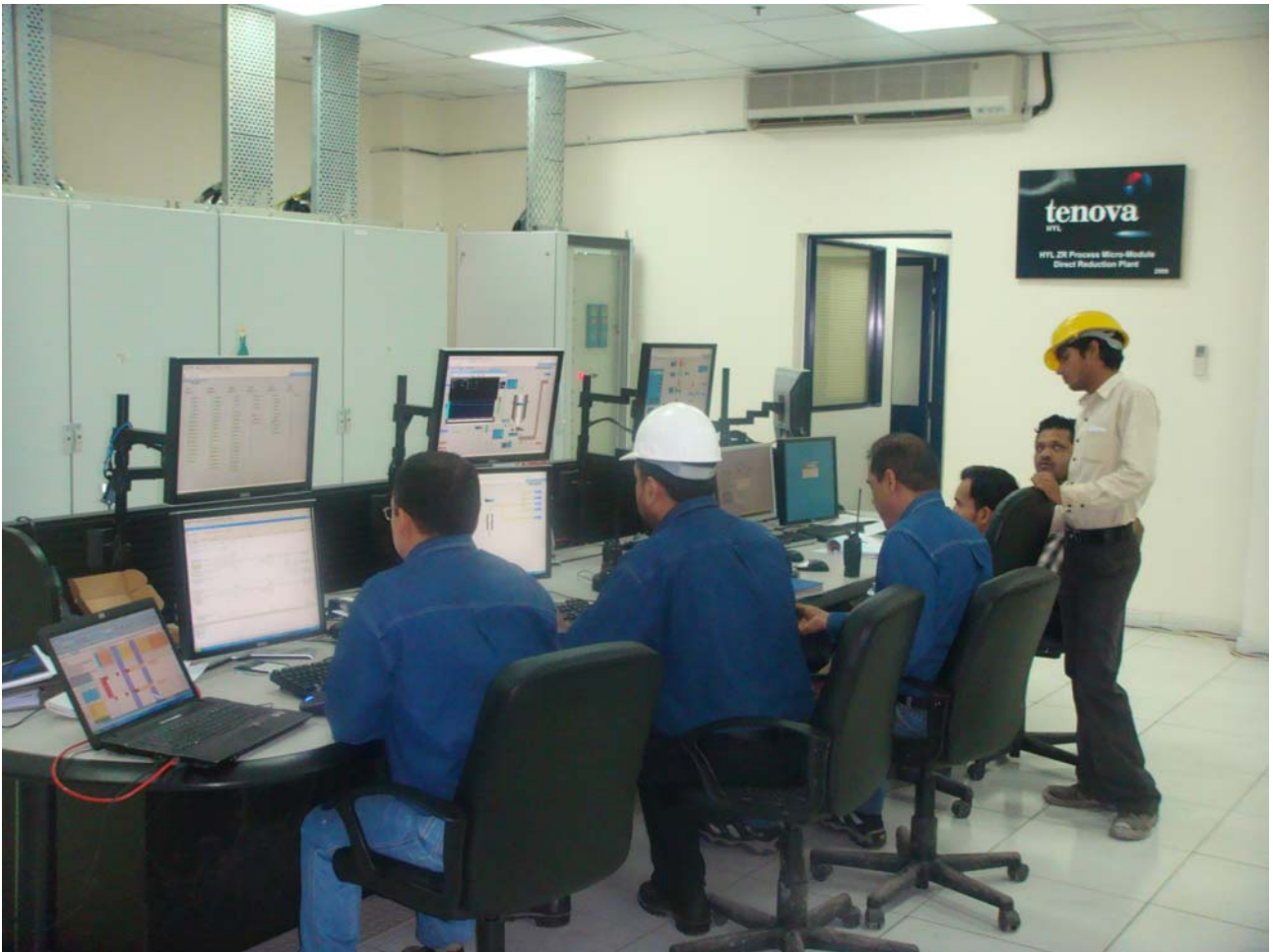
GSPI Micro-Module Control Room
