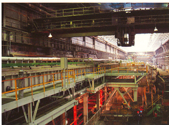
Fig.1 No.1 pickling line
