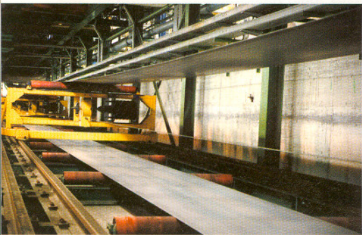
The hybrid push-pull and semi continuous pickling line at Dufenco La Louvière in Belgium supplied by Tenova
