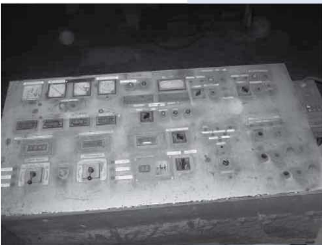
Figure 3. Before the revamp the plant had been in operation for 30 years
