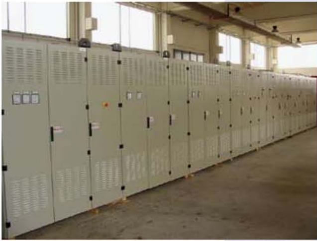
Figure 5. New automation equipment
