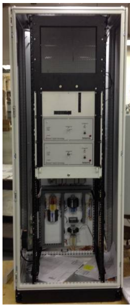
Figure 2 (a). Analyzer Cabinet
