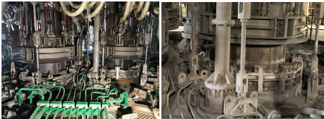
Figure 10. Seal installed on circular AC primary platinum smelting furnace design and supplied by Tenova Pyromet (new and used)
