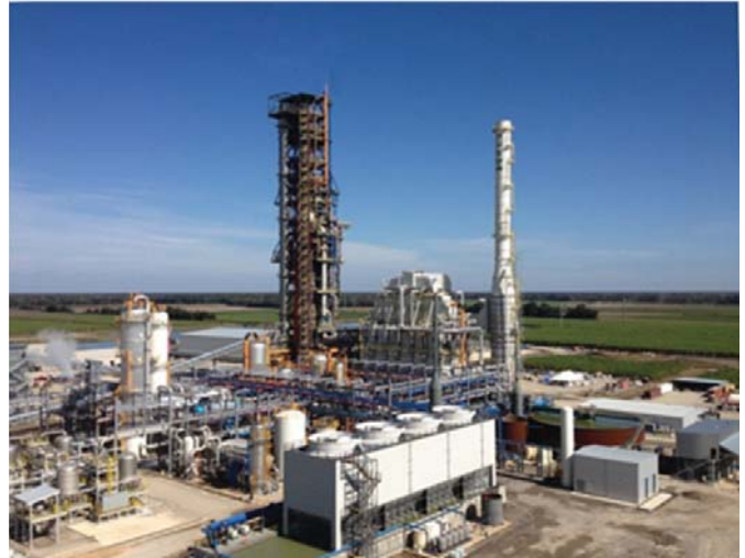
Figure 8. Nucor Steel Louisiana DR plant with CO 2 absorption and sulphur removal system
